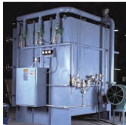
View of a typical gas train.
